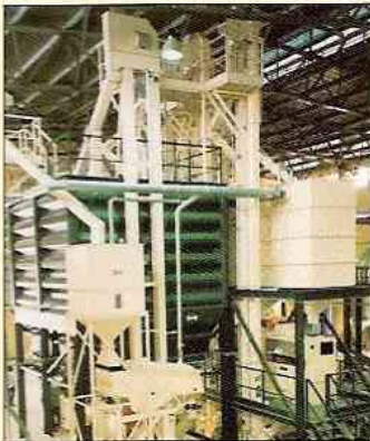
Nga Nam, Soc Trang Province, Vietnam. Integrated Paddy receiving, precleaning, drying and storage plant. Capacity 15 tph including 8 tph complete rice mill.
