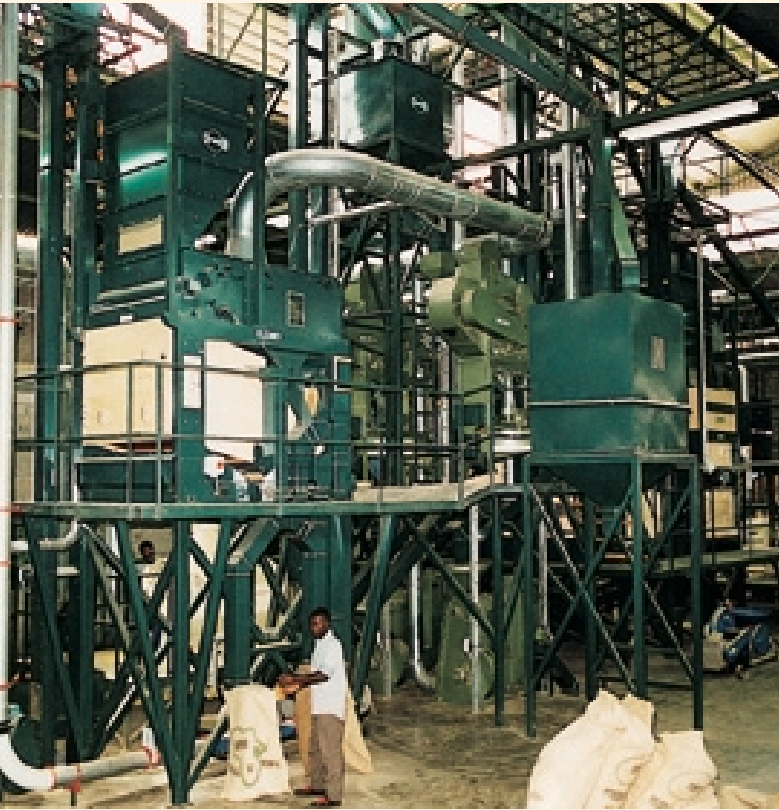
Coffee Processing Plant in Kenya
